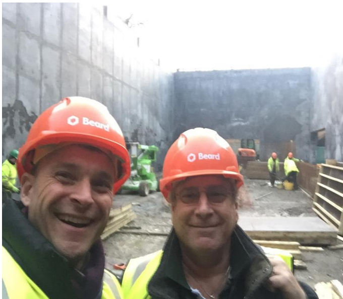
Dan Jones (left), Head Professional, and Peter Luck-Hille (right), inside the Wellington College court, during its erection by Beard Construction (which company also built the Radley court).
